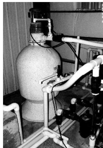
Power wash bead filter on recirculating water system for maturation tanks.
